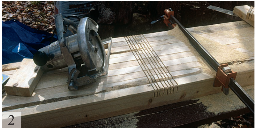
2 Notch the side-wall studs for the 2x4 nailer. Clamp the studs together; then cut 1-1/2-in.-deep kerfs. Remove the waste with a hammer and chisel.
